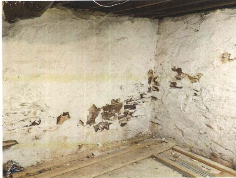
Photograph 1: Parging delaminating from the flagstone foundation wall
