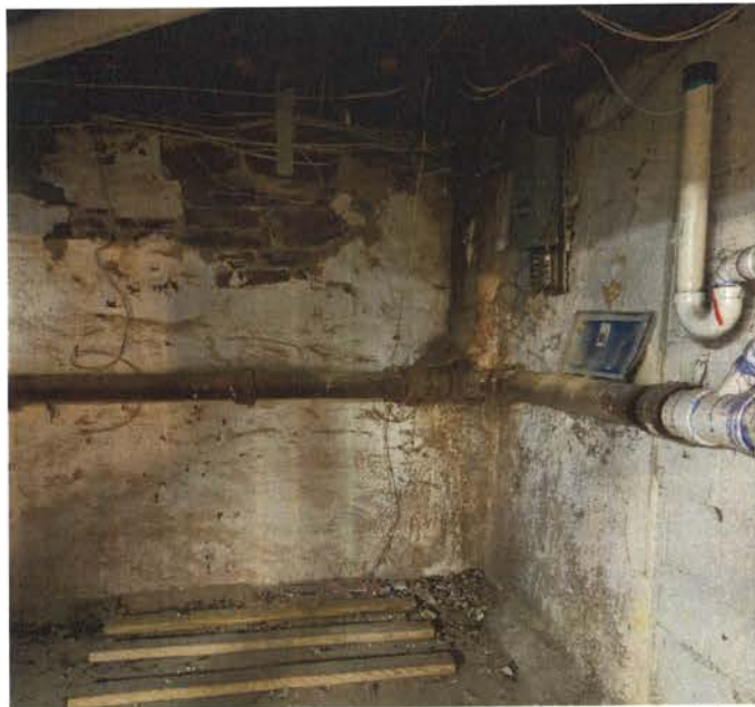
Photograph 2: Signs of water infiltration and parging delamination
