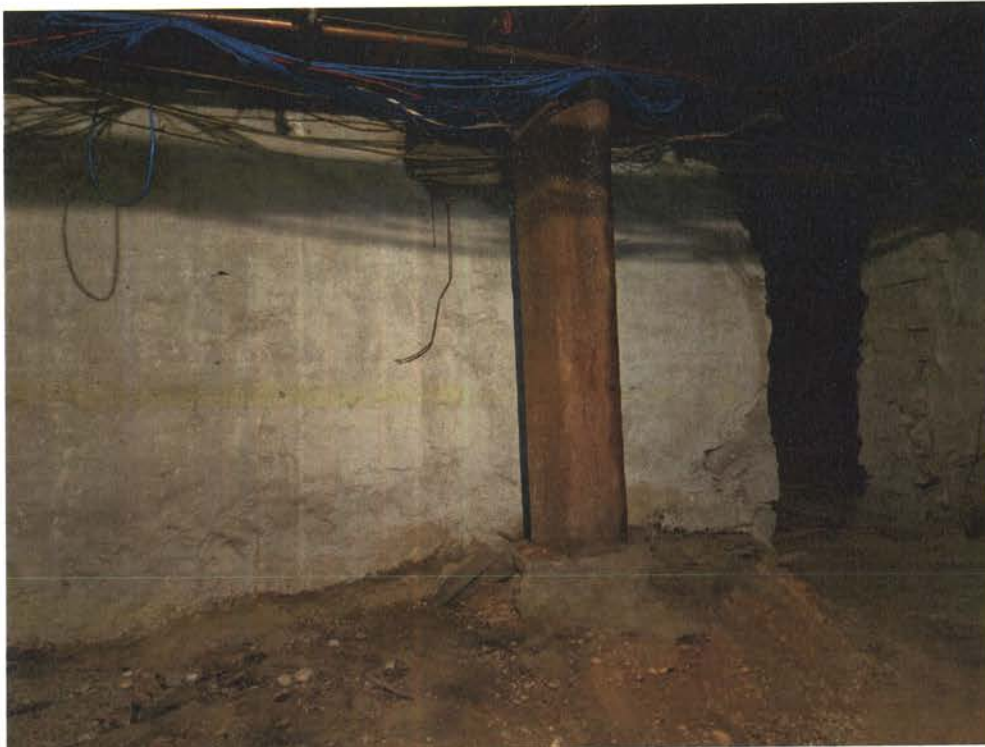
Photograph 7 : Undersized and exposed column footing
