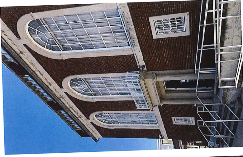
528 STATION AVE • VERTICAL PICKET GUARDRAIL ALONG ROOF • ARCHED WINDOW • RED BRICK FIELD MATERIAL • CAST STONE SIDEWALK BANDING
