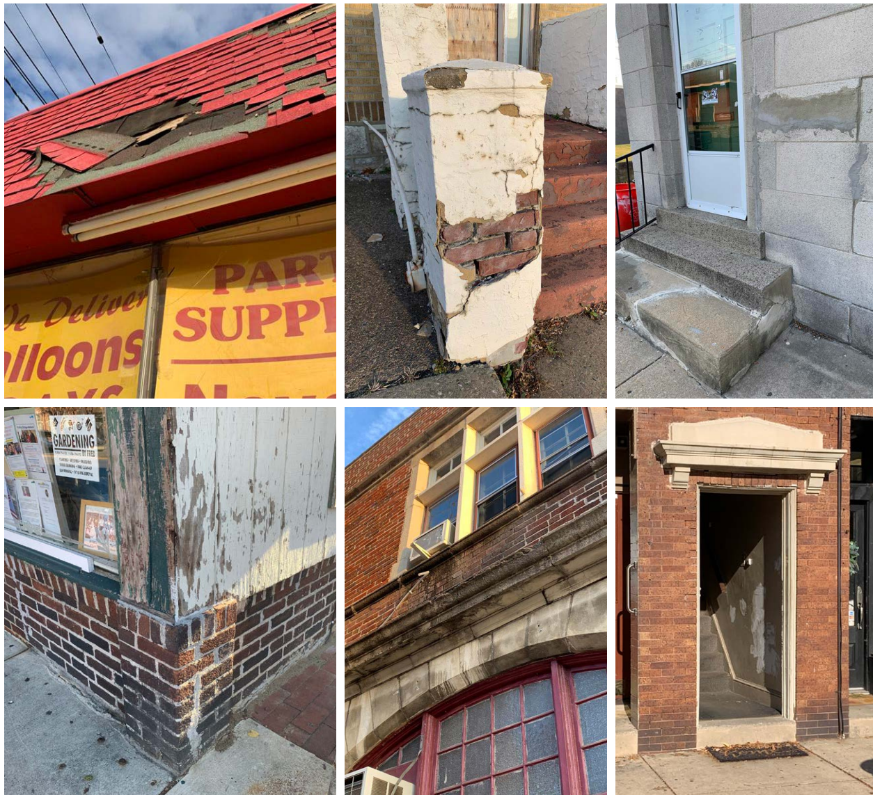
Figure 14. Example of dilapidated building conditions along Station Avenue and Black Horse Pike
